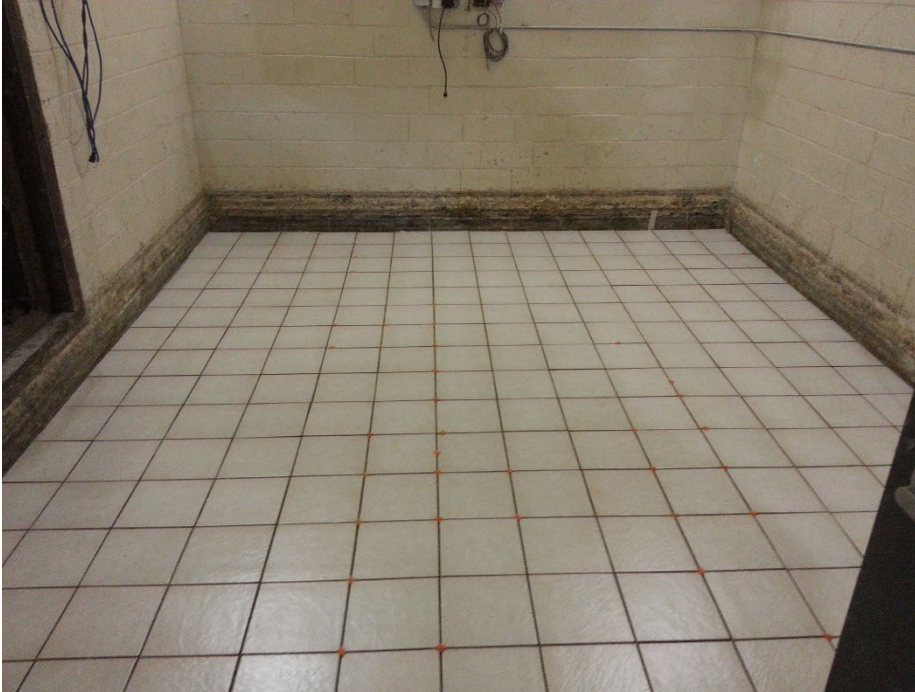
Figure 1 – Specimen mounted on the concrete slab. (Note: spacers were still present at the time the photo was taken, but were removed before installation of grout)
